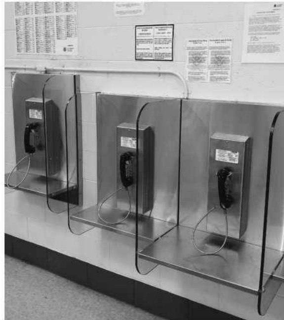
Telephones Provided in Housing Units
